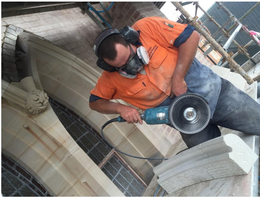
Stone Mason, Tye Murphy from Stone Restorations making the finishing touches to the final piece of stone to be replaced
